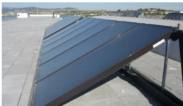
Solar panels on top of many units
